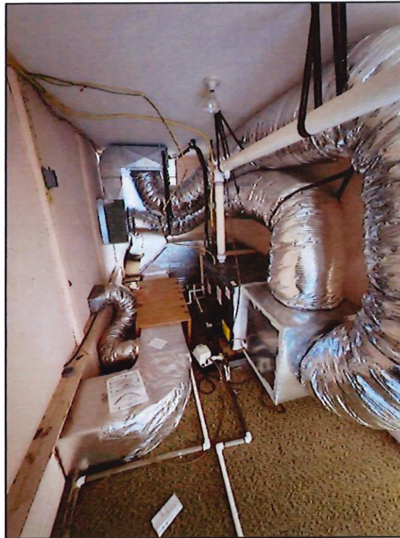
Figure 10. HVAC equipment in the second story.
